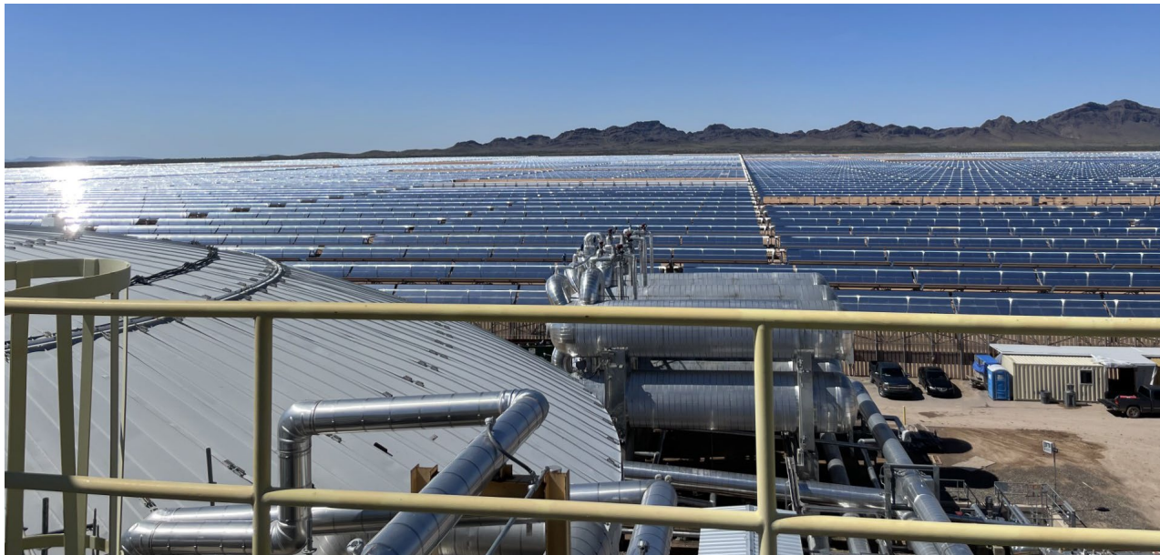
Portion of the Parabolic Troughs used at Solana
